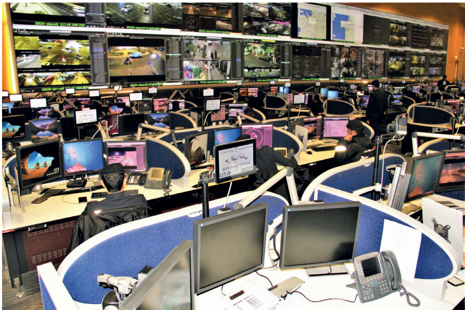
Security surveillance operations room
