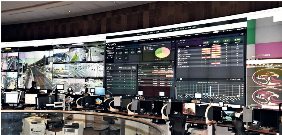
Najm system applications in the command and control room
